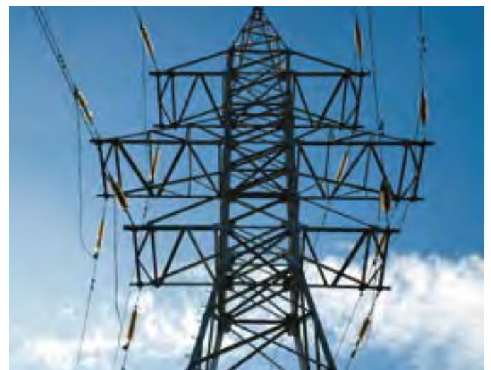
Keep away from high-voltage lines
