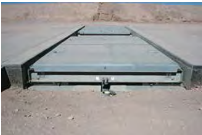
Weighing scales installed
